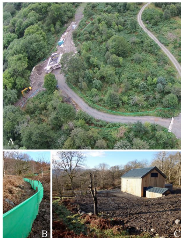
Fig. 2. Loch Lomond hydroelectric development at a site containing high densities of adders ( Vipera berus ) and other reptiles (McInerny, 2016a). (A) Aerial view of the lower section of the construction site, August 2014. This shows the fenced area encompassing the construction site containing the partially built turbine powerhouse, the cleared areas where the underground water pipes had been laid, a movable heavy sheet “gate” placed across the access road, and the intact habitat surrounding the site. (B) Reptile-proof fencing that surrounded the construction site, February 2014; this was ~50 cm high with ~10 cm below the ground. (C) The completed turbine powerhouse, with fencing removed, November 2014. (Photos: C. McInerny)
